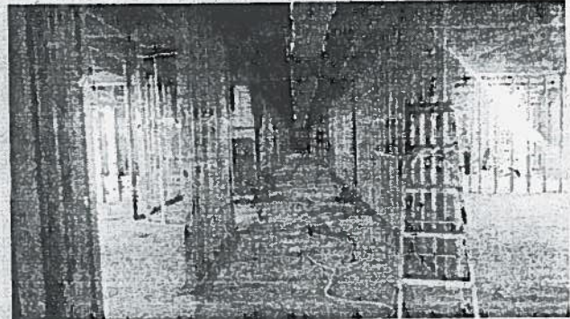
May 21, 2014: wall framing and above ceiling rough-ins begun (new plumbing lines, mechanical ducts, electrical conduits, etc.)
